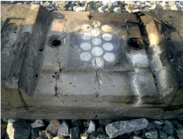
Fig. 11. Cracks in concrete blocks (LVT)
