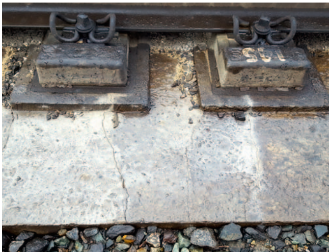
Fig. 2. Cracks in supporting block bed and in concrete slab (Tines)
