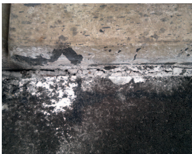
Fig. 10. Leakage from concrete components under the slab (MaxBögl)
