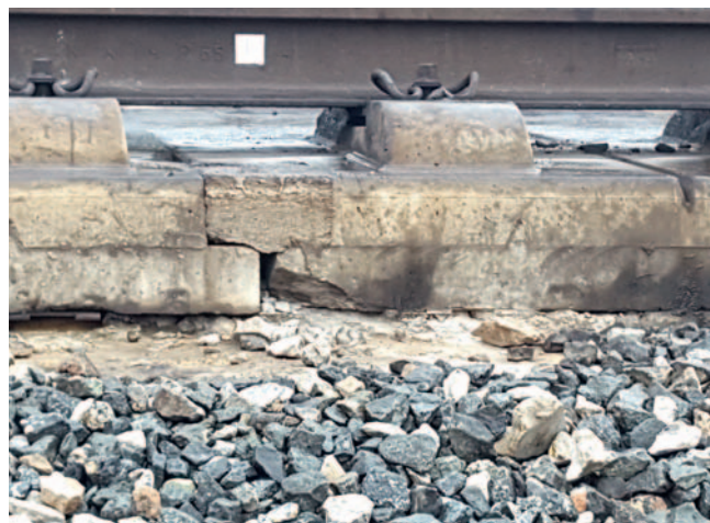
Fig. 9. Slab joint failure (MaxBögl)
