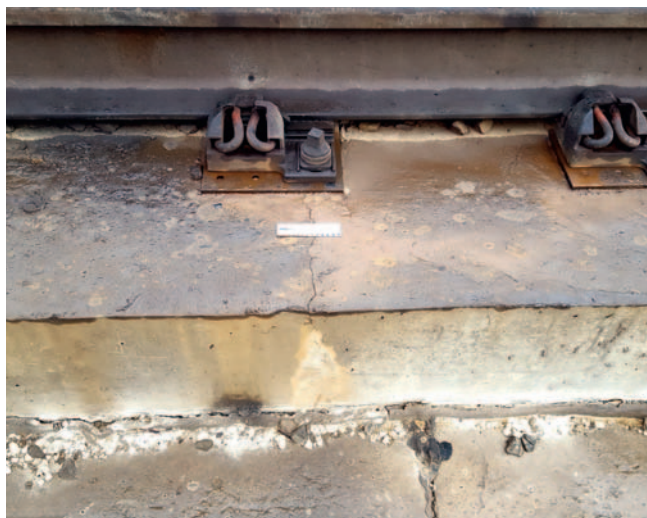
Fig. 6. Cracks in structural slab (Alstom)
