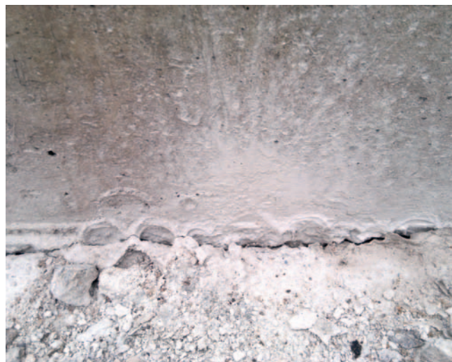
Fig. 7. Leakage of asphalt filler in slab joints (Alstom)
