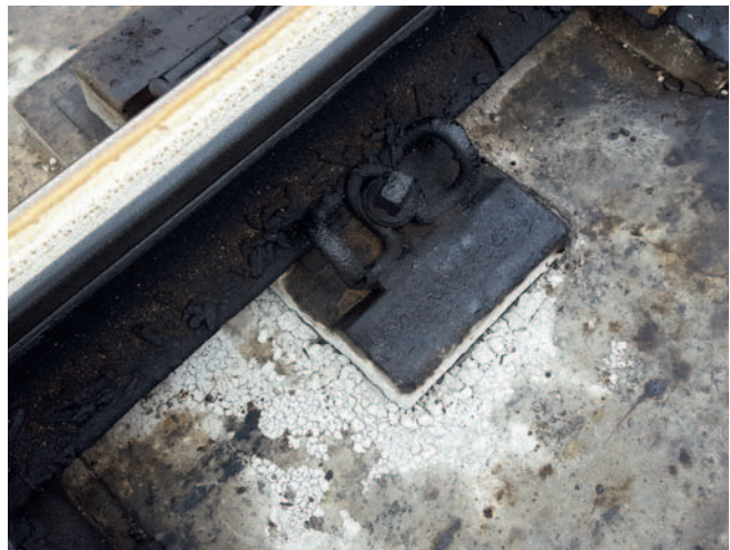
Fig. 3. Loss of grip between supporting blocks and structural slab (Tines)
