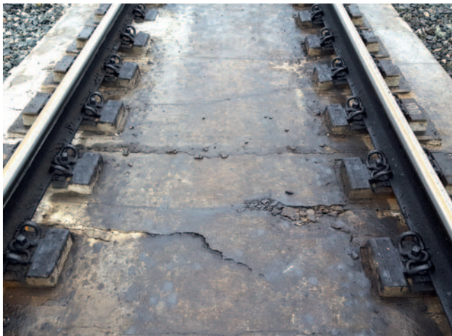
Fig. 4. Full-width fracture of the reinforced slab (Tines)
