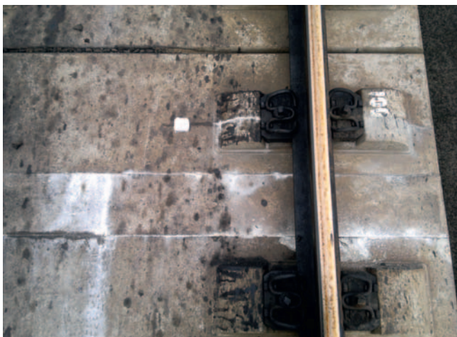
Fig. 8. Cracks in slab and slab joint (MaxBögl)
