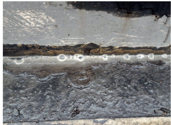
Fig. 14. Cement components bleeding at the joint (LVT)
