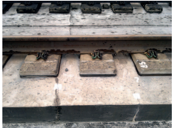
Fig. 12. Cracks in track concrete (LVT)
